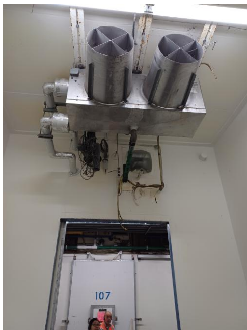
The large fans used in the Stemilt cold stores.
