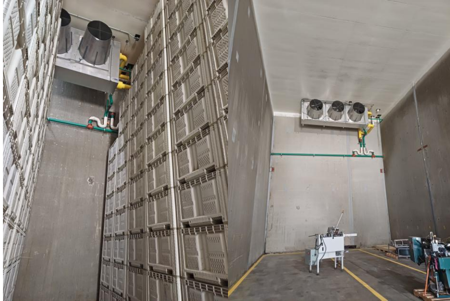
The fans used within the cold rooms for better air distribution.
